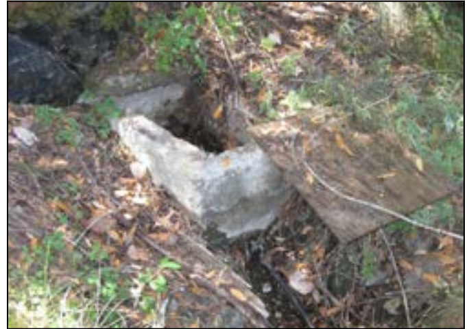
Photo 8. Spring box and irrigation line near Erland Road
